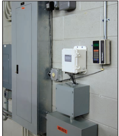
Electricity supplied to the building is sub-metered into dozens of categories that help to identify opportunities to conserve.
