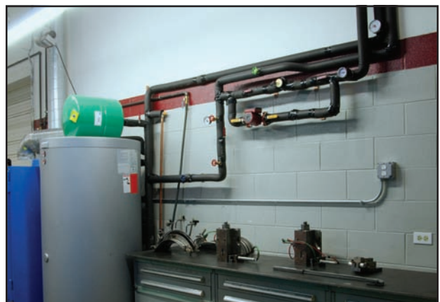
Solar hot water from rooftop collectors is distributed for a variety of uses, summer and winter.
